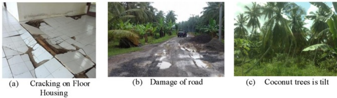
Fig. 4. Direct Impact of Land Subsidence.
