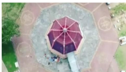
Pagoda Roof (Problem 1)
