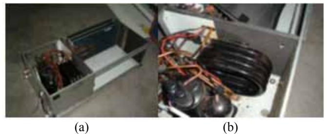
Figure 1: (a) Water Source Heat Pump (b) Condenser Coil
