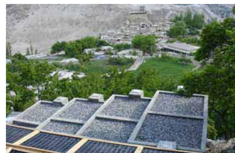
Figure 1 A water filtration system above Altit, in the Northern Areas of Pakistan.
