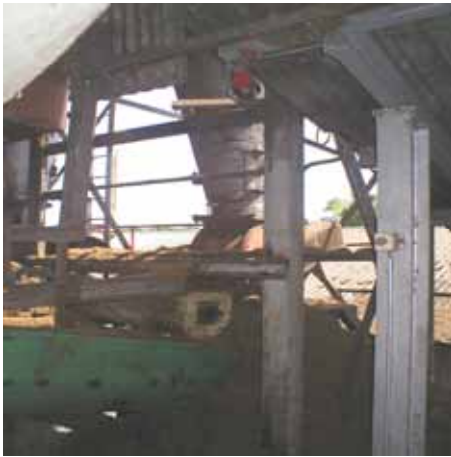
Figure 6: Fiber cyclone, fiber after the separation process use as a boiler fuel
