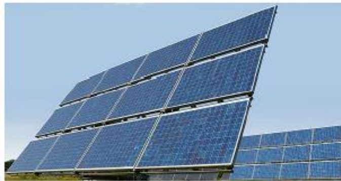
Fig. 2 Series/Parallel combination arrangement of solar PV modules
