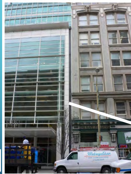
Figure 4. Two buildings separated by a seismic gap covered by a flexible flashing.
