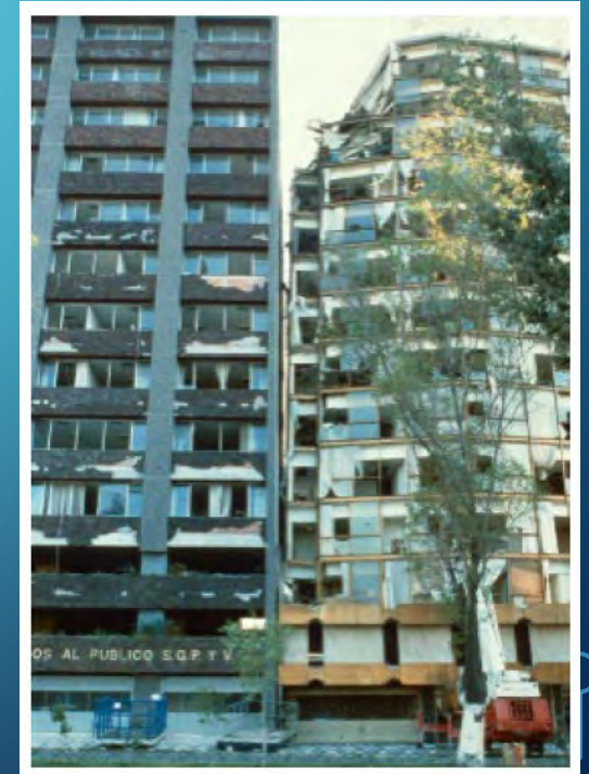
Figure 2. Two buildings have pounded each other with one far more seriously damaged than the other.
