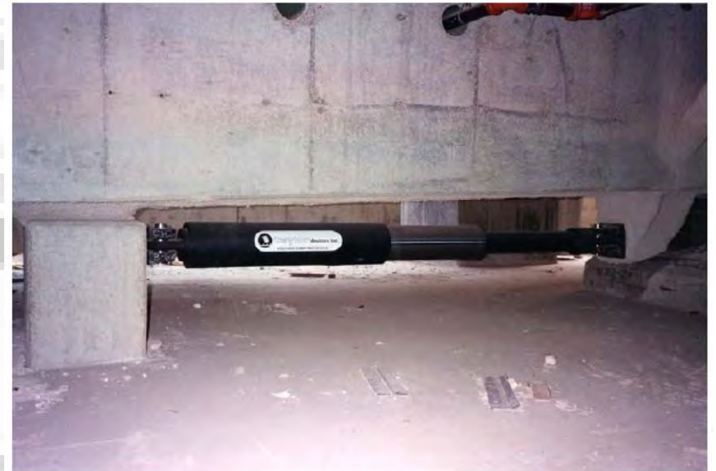
FIGURE 27 ARROWHEAD REGIONAL MEDICAL CENTER INSTALLATION OF DAMPER
