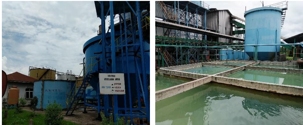
Gambar 4. Water Treatment Plant PMKS PT. SPOI
