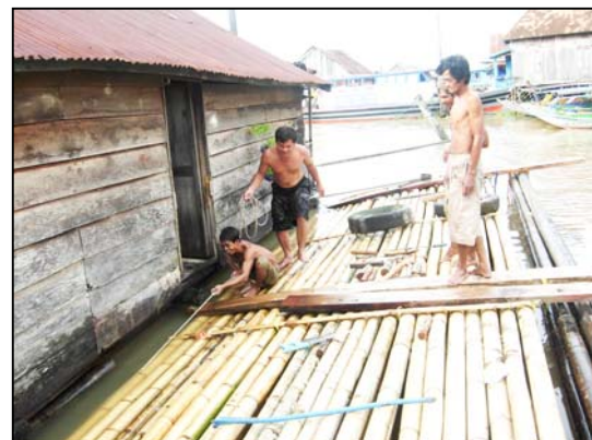
Figure 9. The replacement of the bamboo foundation of raft house.. Source : Field survey, 2007
