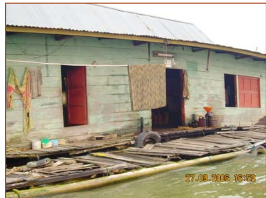
Figure 8. Raft house damaged floor. Source : Field survey, 2007
