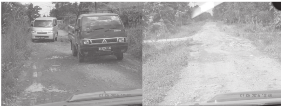
Fig. 2. The condition of rural roads in Tanjung Lago at District of Banyuasin.
