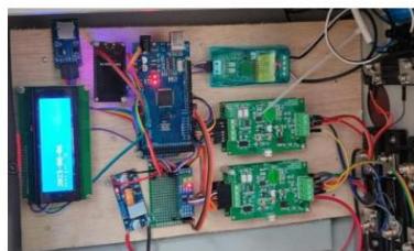
Figure 4. Implementation of IoT in the PV System
