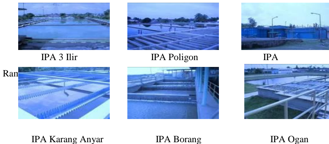
Gambar 4. Instalasi Pengolahan Air (IPA) PDAM Tirta Musi Palembang (Sumber: PDAM Tirta Musi Palembang, 2007)
