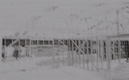
Fig 2 Cold formed steel framing (light steel framing) for residential house in UK (Adopted from Grubb, 2001)
