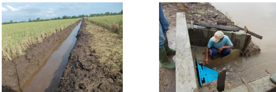
Figure 4. Condition of water level control structures at tertiary channel.
