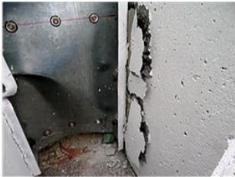
(c) Crushing of concrete
