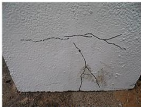
(a) Surface cracks on slab
