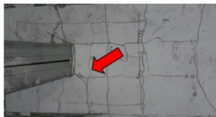
(a) IJT-03 first crack
