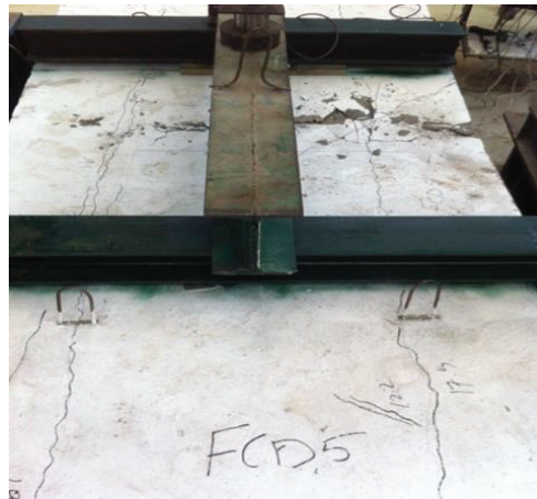
FIGURE 7. Longitudinal crack, CFS thickness 3mm
