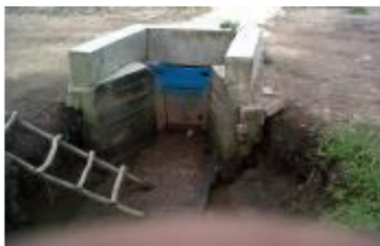
A. Water supply position
