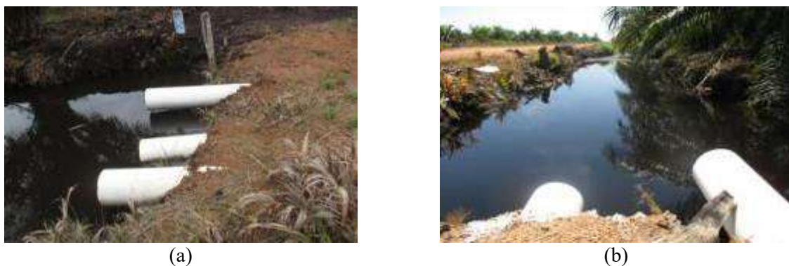
Figure 2. A water-retaining embankment in the secondary channels; in downstream (a) and in the upstream (b) [12].
