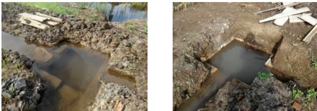
Figure 17. Condition of control box at outfall of tertiary channel
