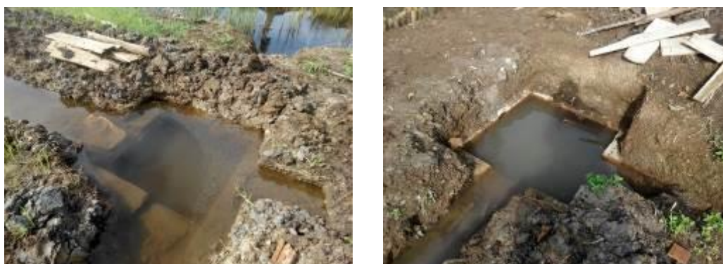
Figure 15. Condition of control box at outfall of tertiary channel
