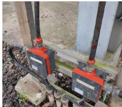
Figure 6 All Junction Box was additionally isolated by red silicon after replacing cable's terminal
