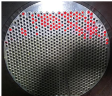
Fig. 2. Deposits of material-clogged SS 304 tubes on the top side
