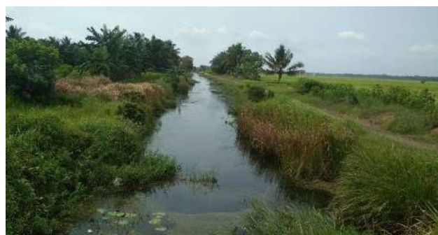
Figure 4. Condition of Secondary P17-6S Channel in 2019
