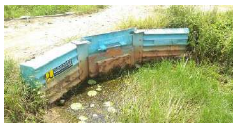
Figure 8. Water gate at Tertiary Channel at TC 7 P17-6S in January (Drainage)
