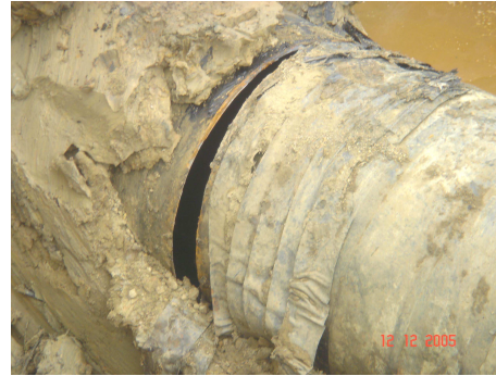
Figure 1. Picture of 42” pipeline rupture in weld joint area.
