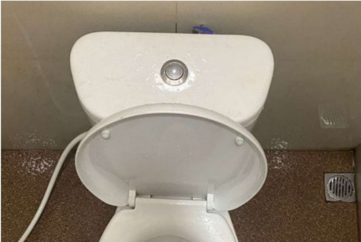
Gambar 4. 15 Toilet one flush
