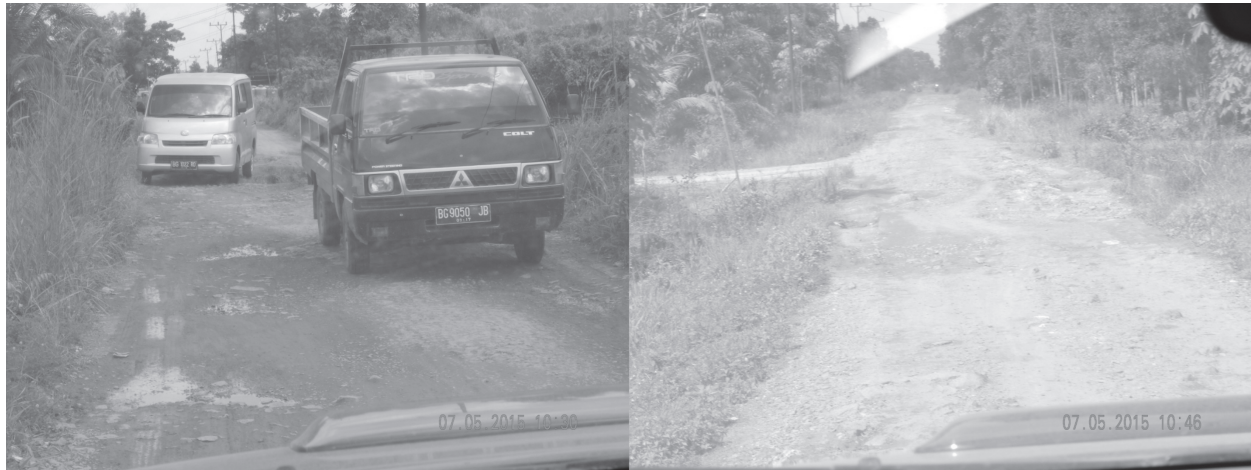
Fig. 2. The condition of rural roads in Tanjung Lago at District of Banyuasin.
