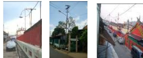
Picture 13. Electricity in Kampung Cina
