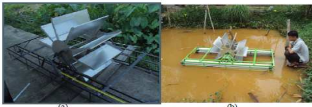
Figure 3: (a) The wheel and supporting frame in construction. (b) The floating test is conducted with PVC pipes at the left and right sides.
