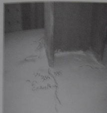
Figure 19. Crack on concrete slab.
