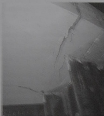
Figure 20. Failure due to cracks on concrete slab.
