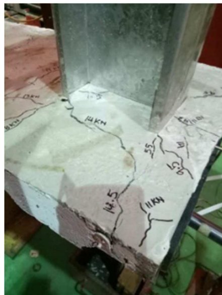
Figure 9. Cracking near to the column in tension zone
