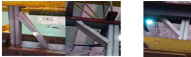
Figure 4. Failure on wall panel haunches
