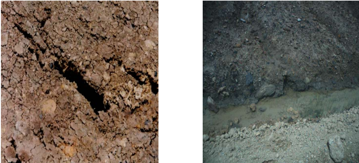
Figure 3 Signs of distress at fill surface prior to landslides
