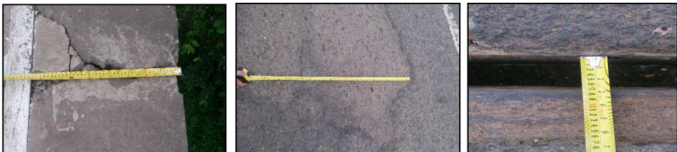
Fig. 2. Damage measurement on truss bridge.
