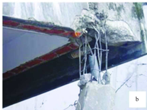
FIGURE 10. Bengkulu Earthquake in 2007, a). The collapsed shophouses, b). Planting utility pipes in the column (source: Boen 2007a).
