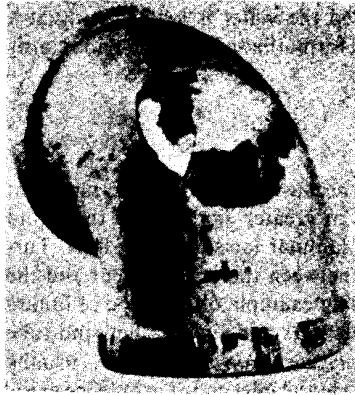
Figure 3-45 Impingement in steam condensate line.
