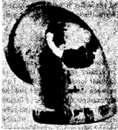
Figure 3-45 Impingement in steam condensate line.
