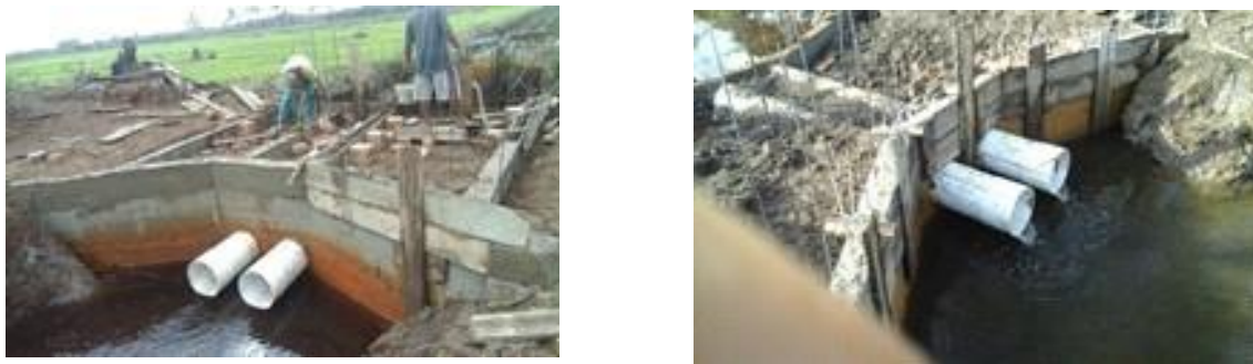
Figure 5. Hydraulic structure in tertiary canal for water retention and control drainage in tidal lowland type C.
