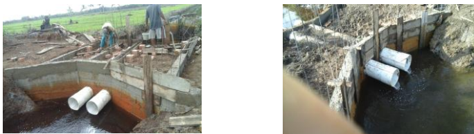
Figure 5. Hydraulic structure in tertiary canal for water retention and control drainage in tidal lowland type C.
