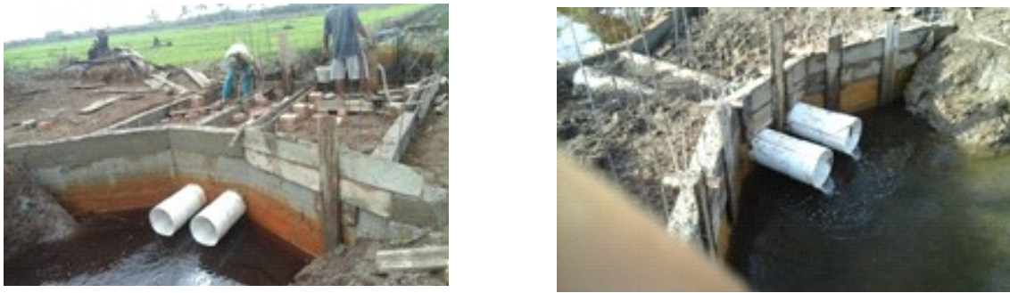
Figure 5. Hydraulic structure in tertiary canal for water retention and control drainage in tidal lowland type C.
