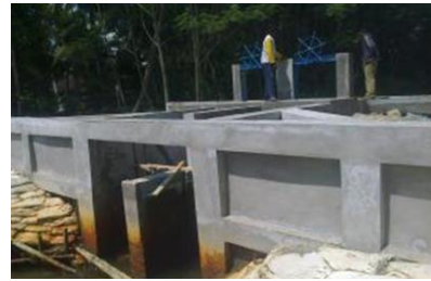
B. Secondary gate
