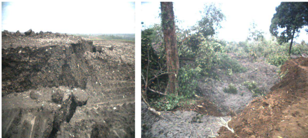
a. Tension crack at the crest of failure
