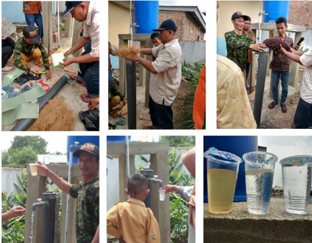
Figure 9. Installation of swamp water filtration and the filtered water has been produced.
